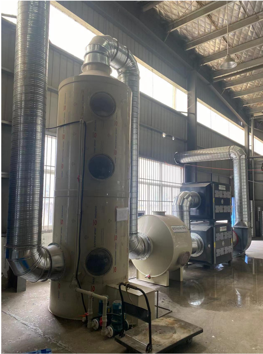
喷淋塔+二级活性炭处 理+15m 高排气筒 DA002
